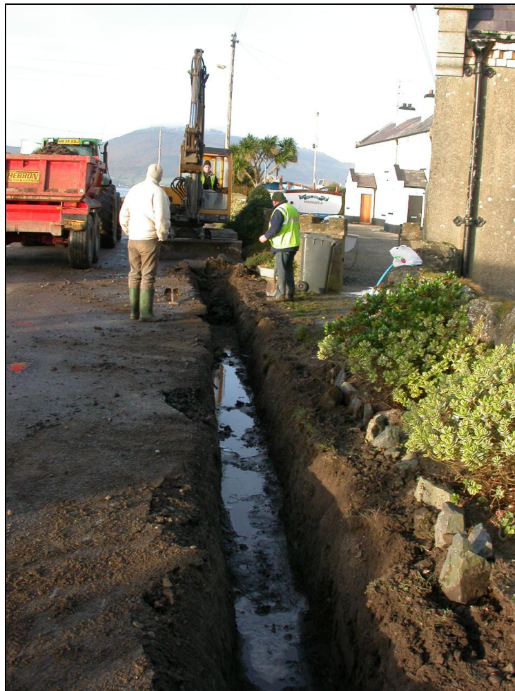
Plate One: Monitoring of the mechanical excavation of Trench One in progress (looking west)
