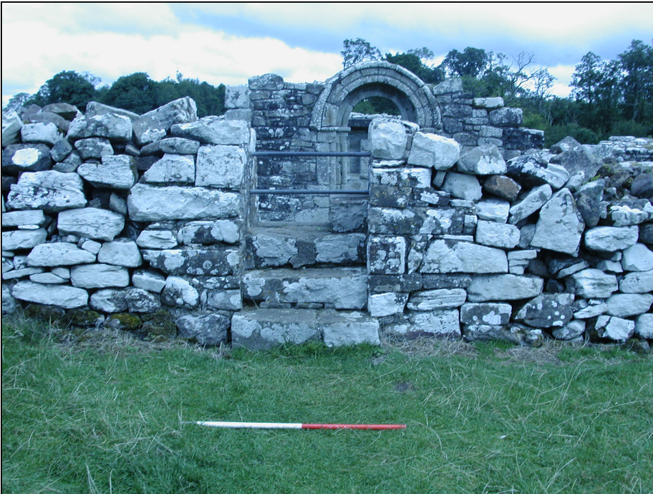
Plate 2. The entrance stile at White Island church, prior to the installation of the handrails. The 12 th century Romanesque doorway is visible in the background (facing north).
