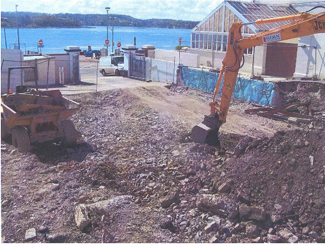
Plate Three: Phase Two mechanical excavation of the development site, looking south-west.
