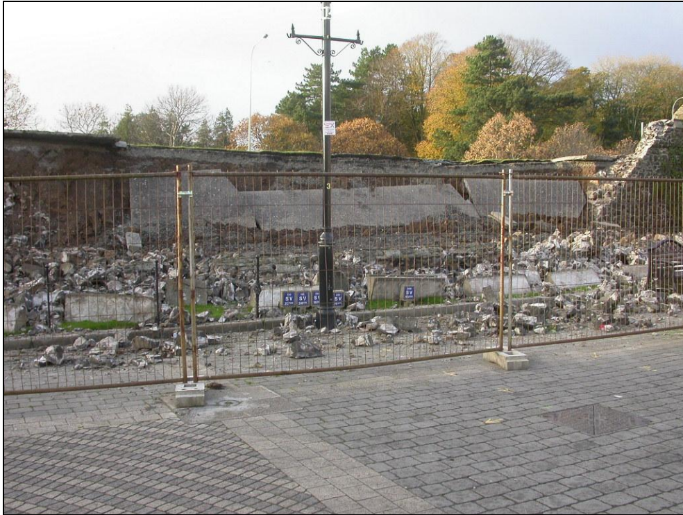
Plate 1: View of collapsed section of bastion wall, looking north-east from Market Square
