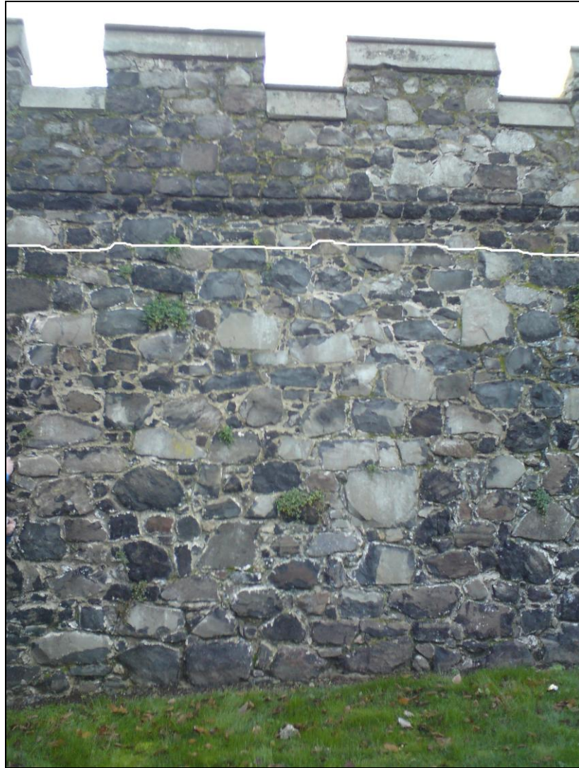
Plate 4: Upstanding section of bastion wall prior to dismantling. Line separates 19 th -Century additions, including corbelling and parapet, from the earlier bastion wall below
