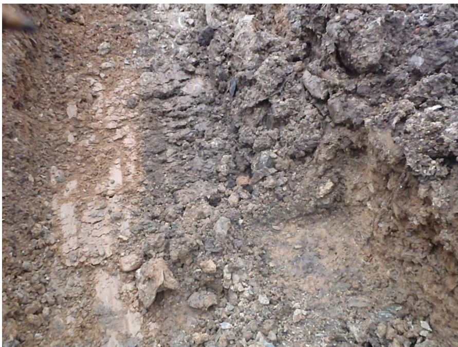
Plate 33 Southwest facing view of fourth foundation cut, post removal of section of wall which encroached on new extension foundations
