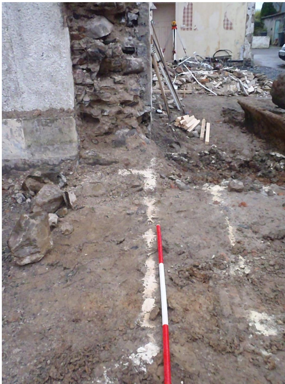
Plate 28 Northwest view of arbitrary edge of brick floor created by prior removal of original cross-wall, within the third foundation cut, pre-excavation of foundations.
