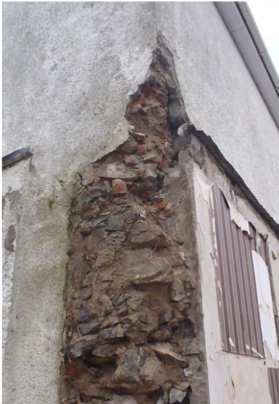
Plate 14 Northwest facing view of corner of Inishargy House post removal of the cross wall
