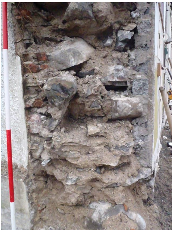
Plate 13 Northwest facing view of corner of Inishargy House post removal of the cross wall
