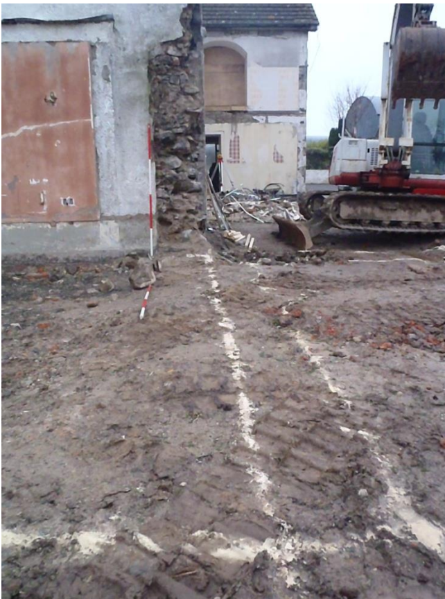
Plate 27 Northwest facing view of third foundation cut, pre-excitation, along the line of the now removed cross wall
