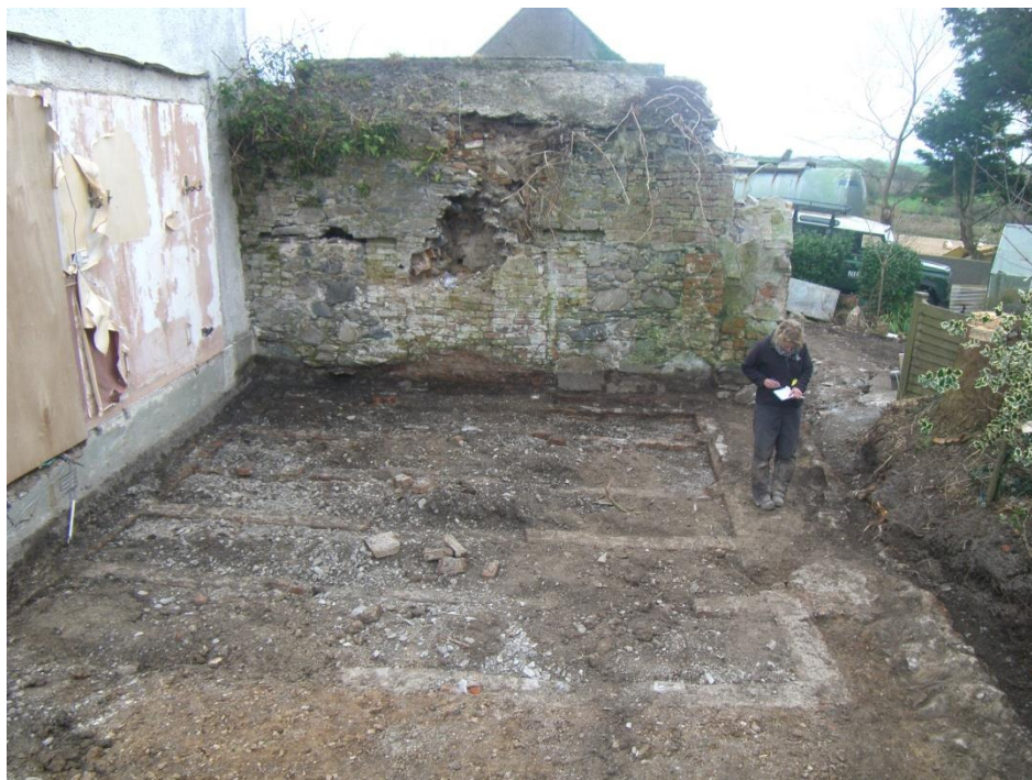
Plate 17 Northeast facing view of cross wall and brick walls uncovered during evaluation
