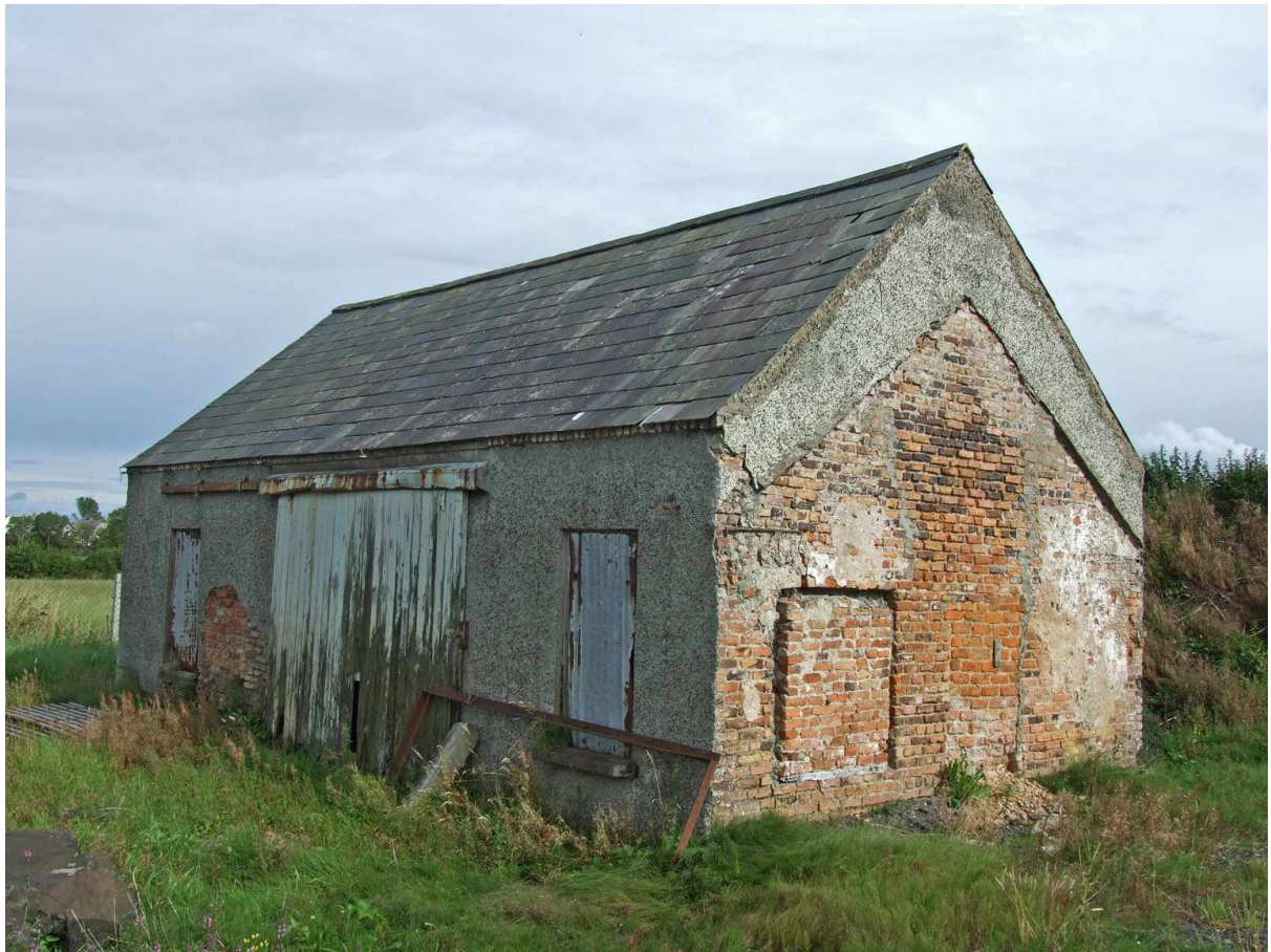
Photo 1: View of north wall of house and west gable (photo courtesy of Paul Logue, NIEA)
