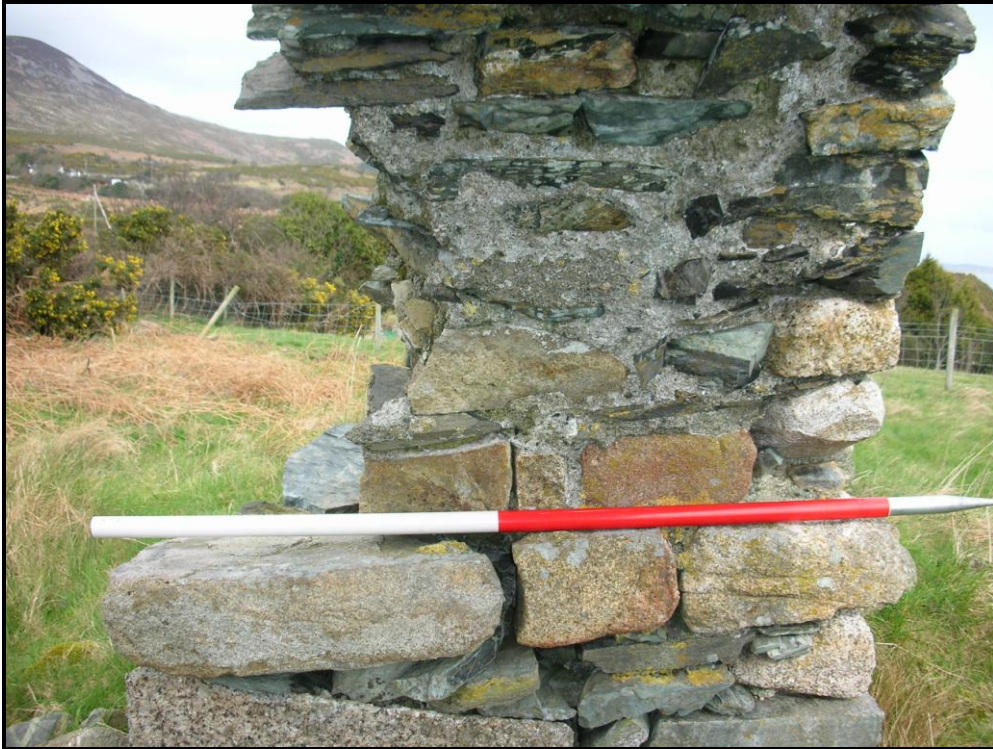
Figure 23: Loss of supporting stonework from the chancel arch, looking north
