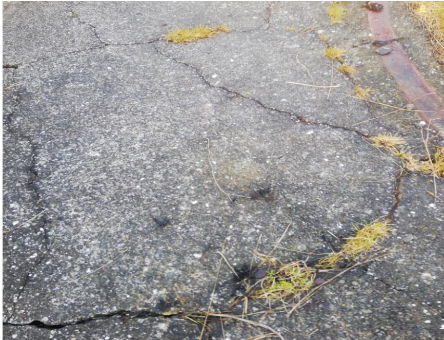
Fig 17 Cracks on the concrete circular platform for the summer house near the iron rail
