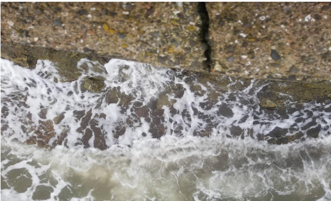
Fig 28 Waves covering the base on a normal tide.
