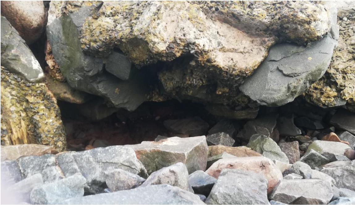
Fig27 Undermining at the east side of the skirt. The eastern side of the base skirt is in similar condition to the west side.
