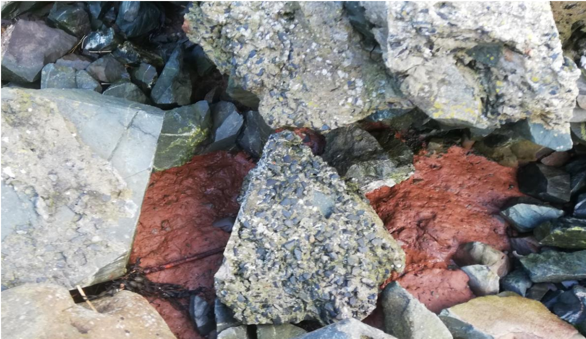
Fig 25 the concrete on the triangular stone is the same as on the adjacent stones on the surface of the skirt, showing that everything from below the surface of the skirt to the clay layer has been washed out.
