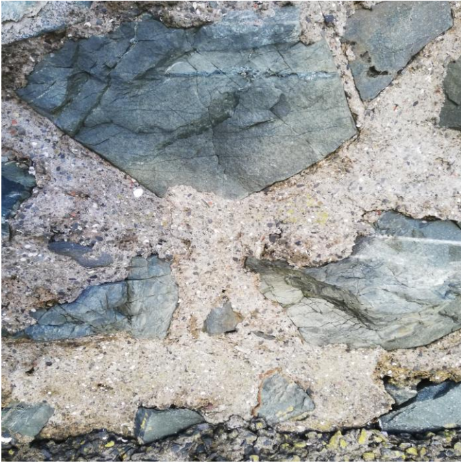
Fig 21 Patched grey stone work, patches at different times
