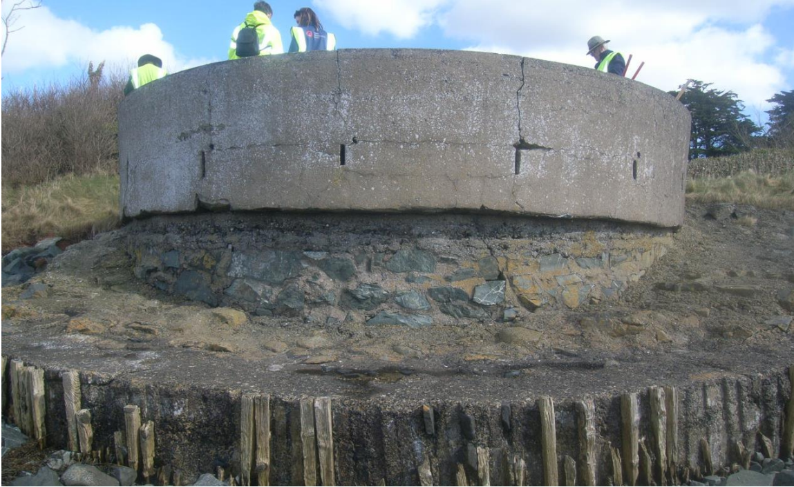
Fig13 Summer house from the beach, the base, the protective wall and the foundation.
