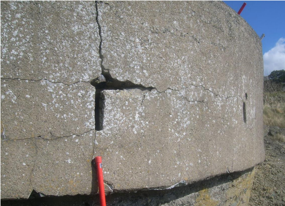
Fig16 Cracks going three ways, vertical and horizontal. The horizontal cracks follow the junction of the protective wall and the platform.
