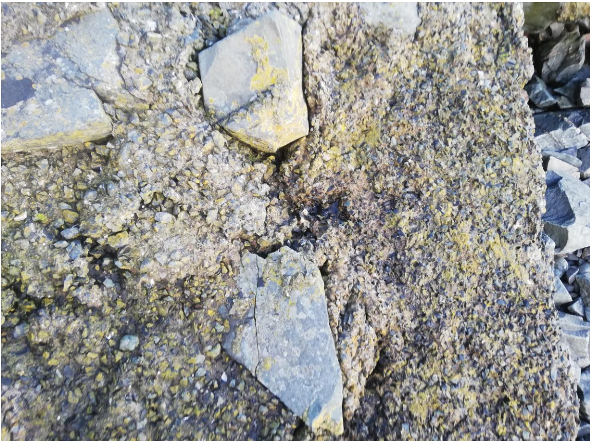
Fig 20 three different concrete mixes on top of base skirt. Note the crack in the stone at the bottom of the picture.
