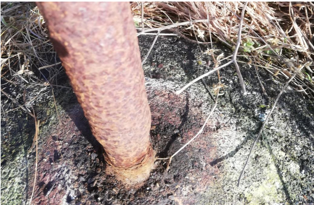
Fig 12 Close up of the base of the axle showing corrosion
