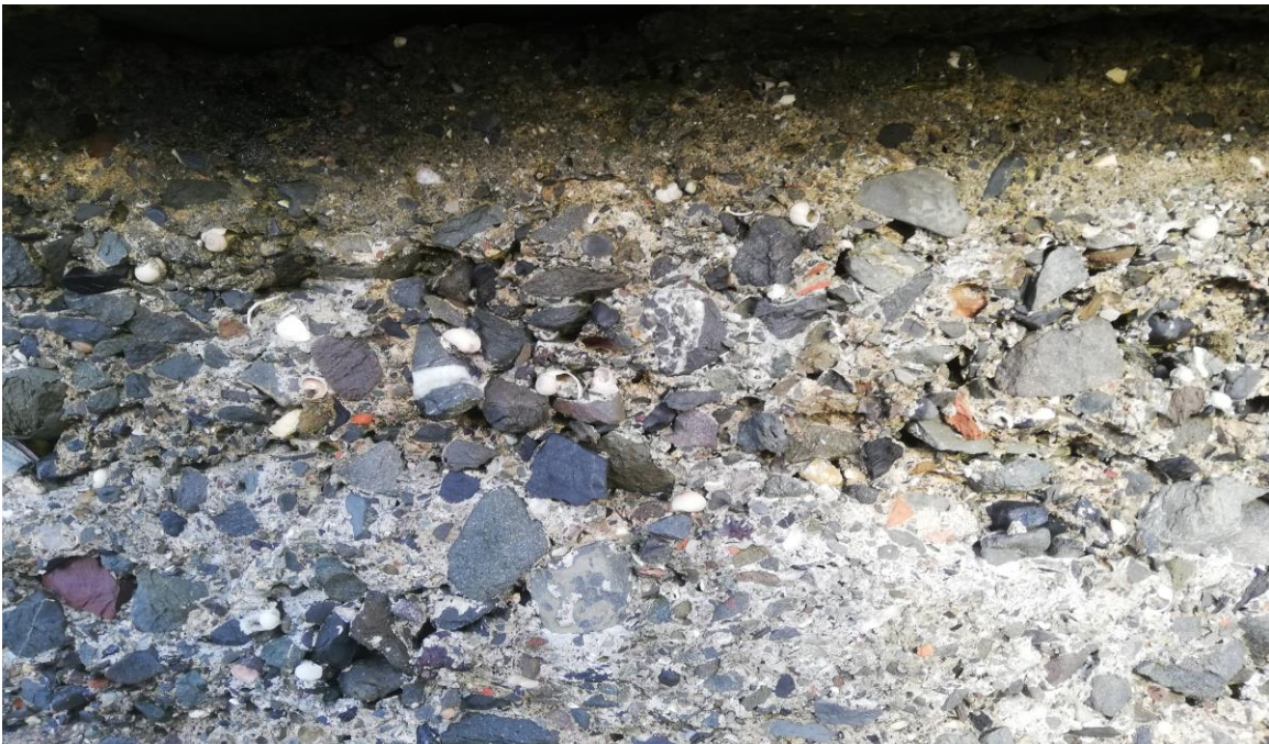
Fig 22 Close up of base, three different concrete mixes, very poor quality aggregate including seashells.
