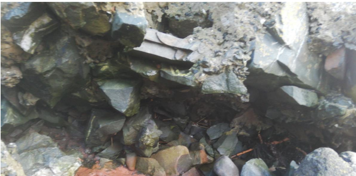
Fig 26 More undermining of the base, east of Fig 24
