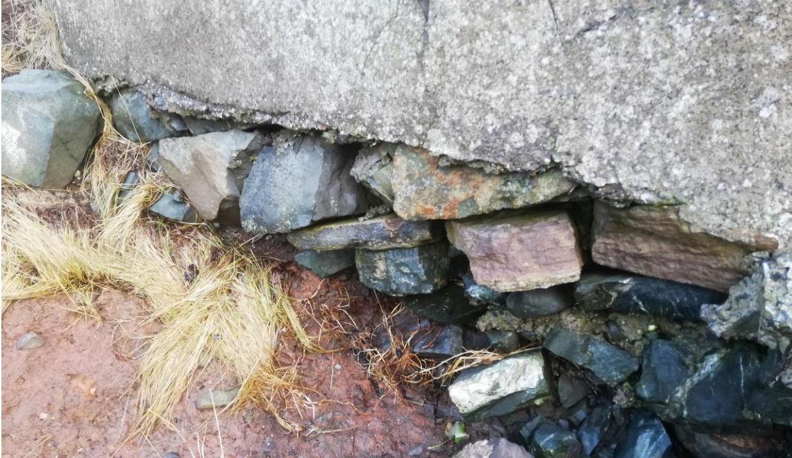
Fig 23 close up of packed stone filling a gap at the clay bank, where the base has been undermined.
