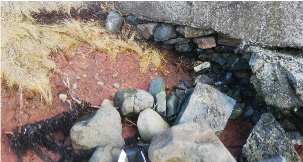
Fig24 Red clay exposed, which had been covered by the skirt.
