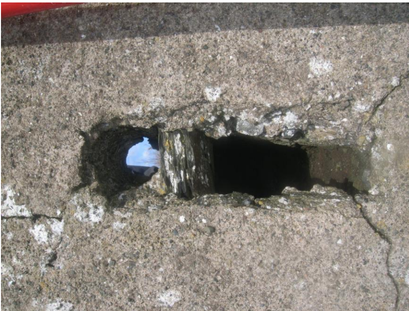
Fig14 Hole in the wall showing cracks going right through the wall.
