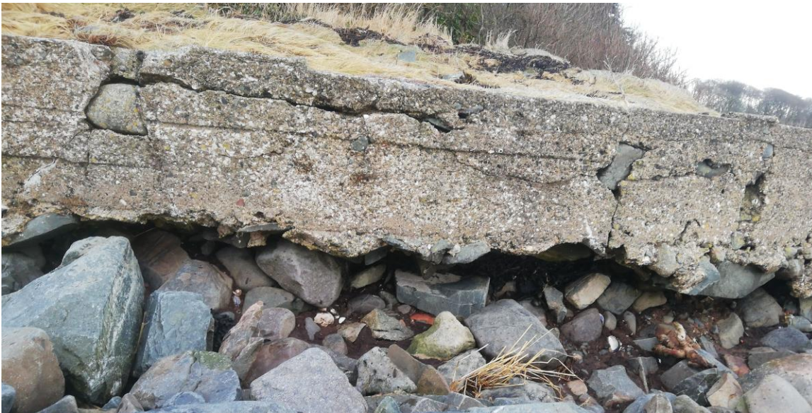
Fig 30 Undermining of the base of second summer house
