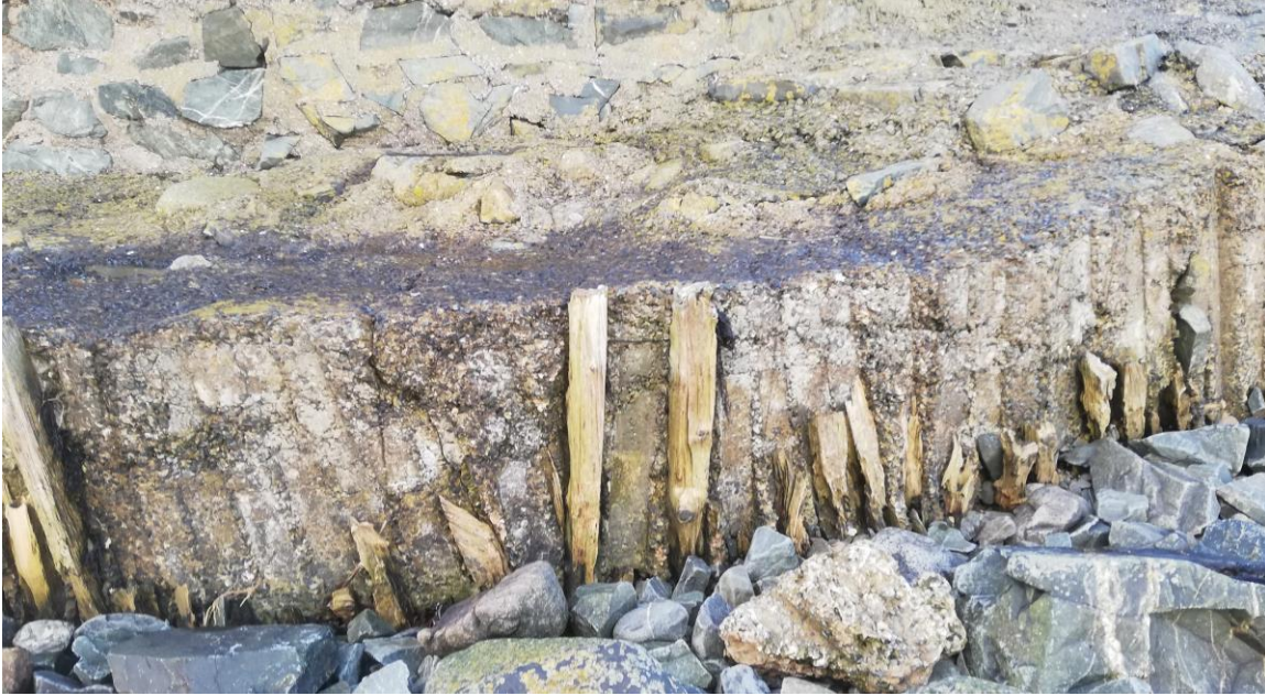
Fig 19 remains of wooden shuttering at the bottom of the base. Again note the layers of different concrete
